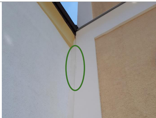
West; Kirche-Turm; örtlicher Riss in Fries
